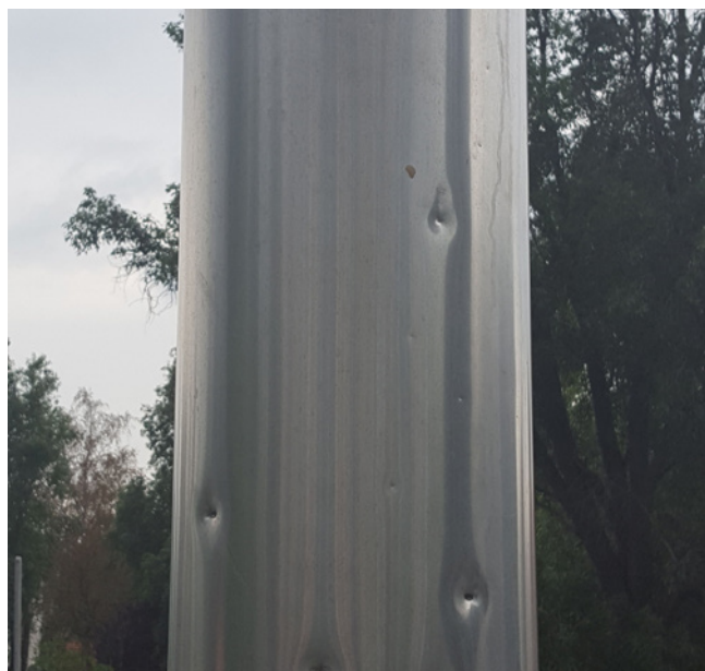
Fig. A. Damage of the chimney surface
