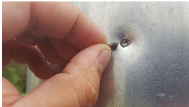
Fig. B. Damage of the chimney surface
